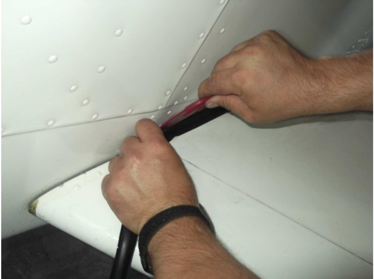
Working the bulb of the seal into the gap with a plastic putty knife. Tough, inch-by-inch work with plenty of Miracle Bubbles soap.
