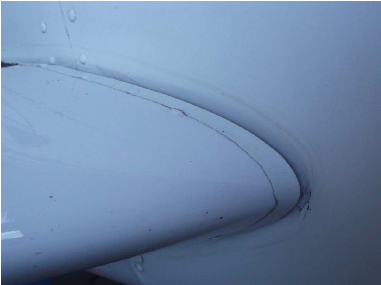
Paint line dates the seals to before the last paint job 25 years ago.
