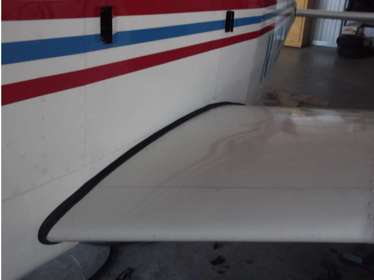
New seals installed, looking' good, now I can finally wash and wax my wing roots normally.
